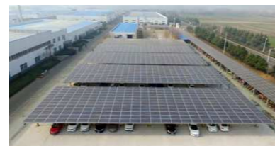
东海基地车棚分布式项目 Carport Distributed Project in Donghai Manufacturing Base
