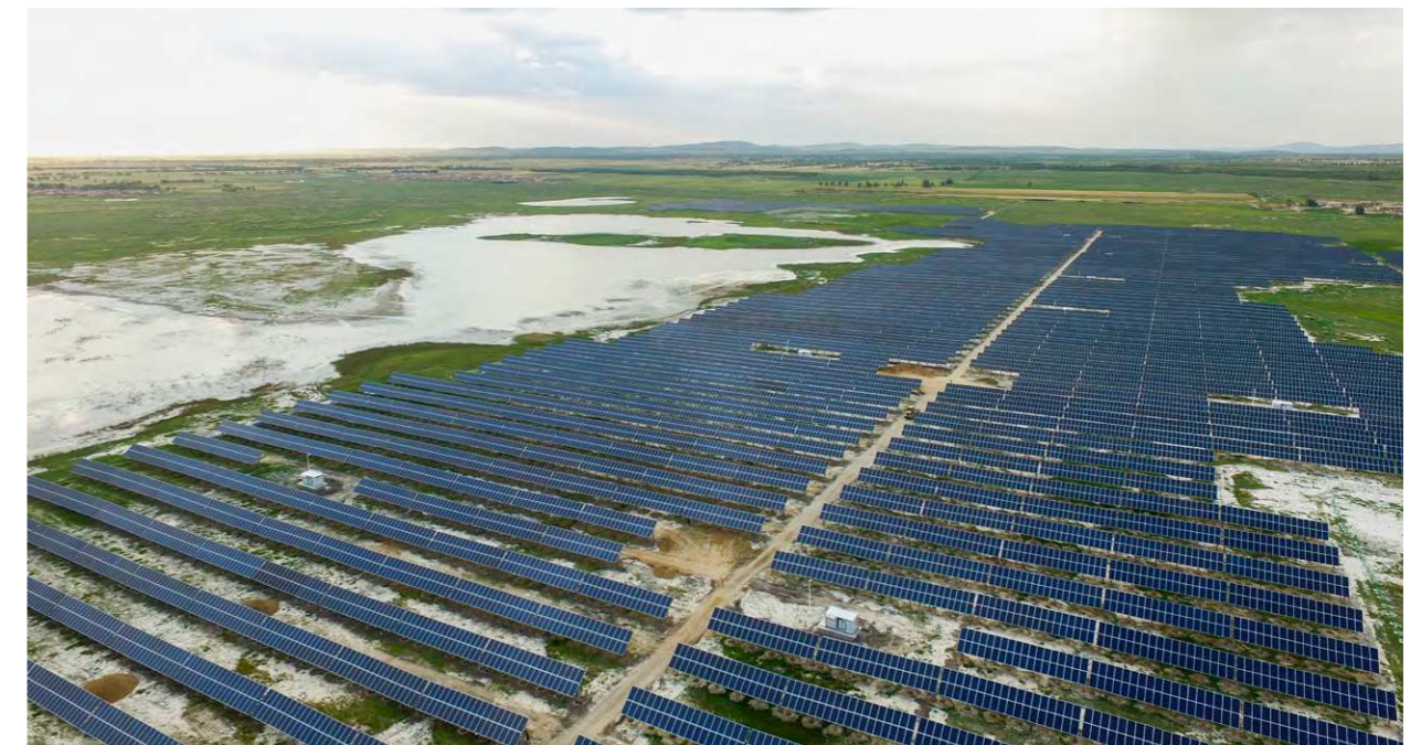
晶澳河北康保20MW光伏扶贫电站 JA Solar's photovoltaic poverty alleviation power station in Kangbao, Hebei Province (20MW)
